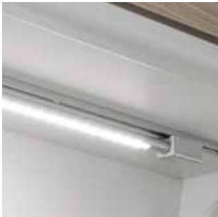
Energy-efficient LED interior lighting.
